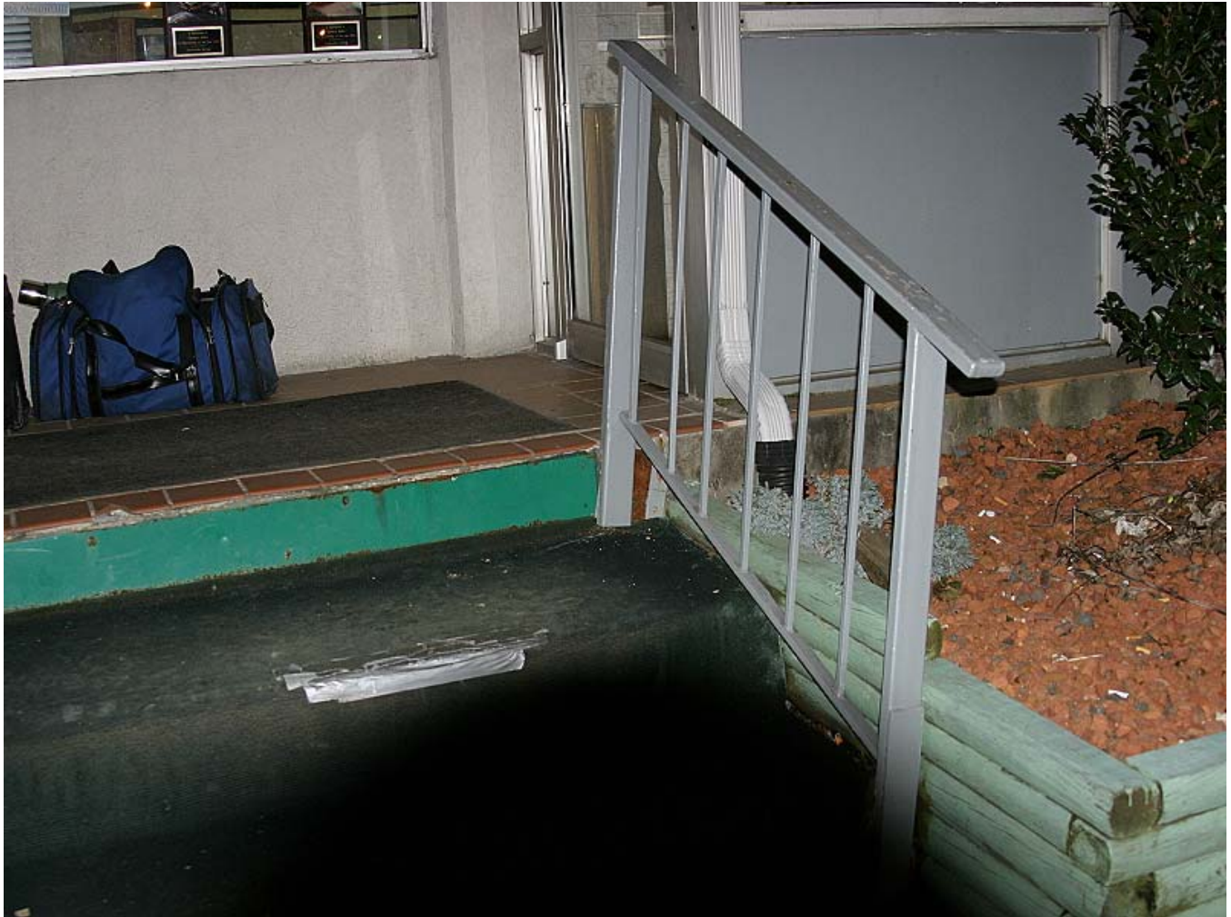
View of North side entrance to main lobby of motel. The upper / top portion of the South banister / railing is not secured with bolts and is loose. Outdoor carpeting repair made with duct tape.
