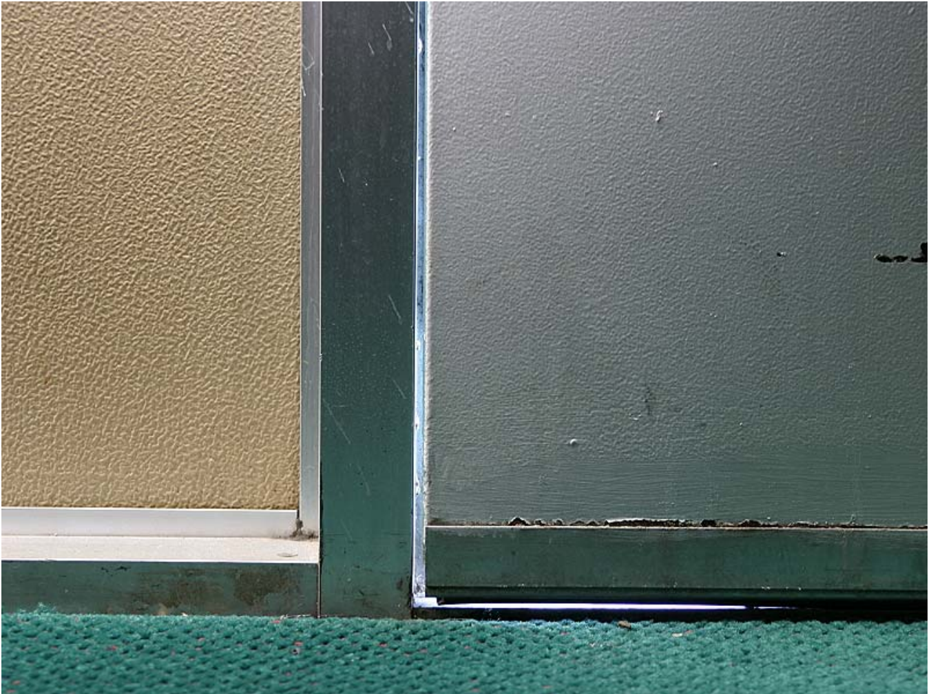
Many of the rooms have cracks around the door casing which allow light and air to seep in to the rooms.
