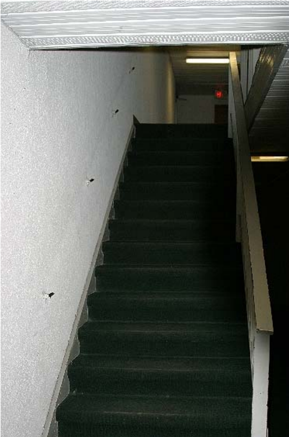
Image of stairway from first to second floor interior corridor which shows railing / banister removed from left wall and the remaining bolts (to which the railing was attached) covered in electrical tape.
